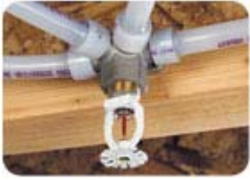
A typical network fire sprinkler installation using PEX tubing. The tee is installed to provide a connection to the plumbing fixture(s) within the dwelling. Photo courtesy of Uponor.
